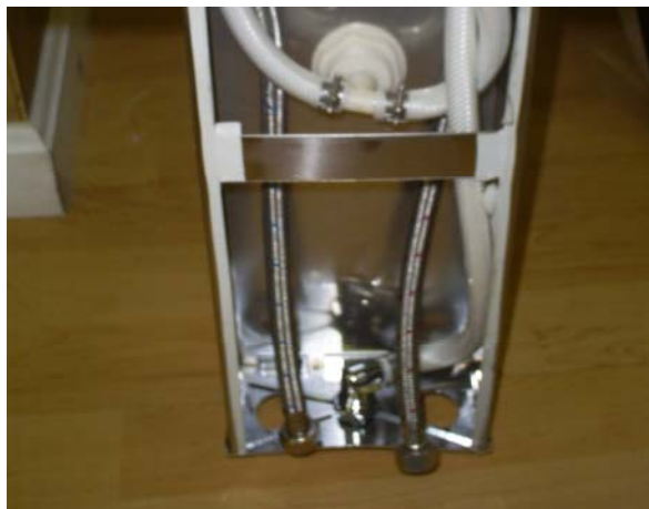
Cold & Hot Pipes
